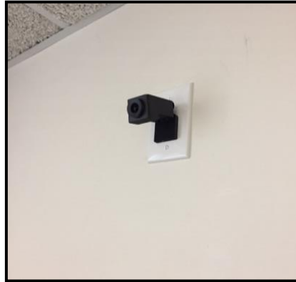
Figure 2: Camera mounted on south wall of room
